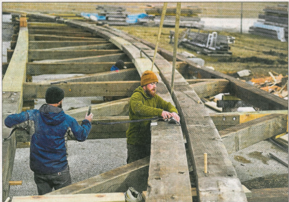
Timber framers Jake Kern, left, and Will Johnson work on the restoration of the Dreibelbis Station Covered Bridge at Lancaster County Timber Frames Inc. in York County.
