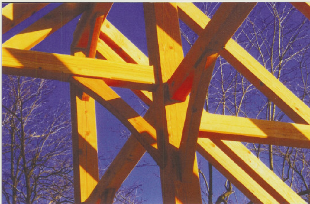
This Manheim area house, under construction, is a combination of conventional framing and timber framing.
