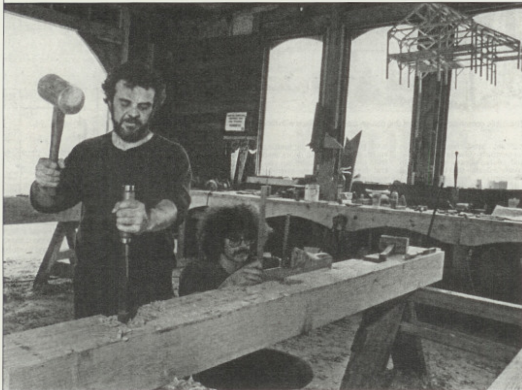
Timber framers Tony Zaya, left, and Bruce Simmons, are preparing two timbers for donation to the Habitat project.
