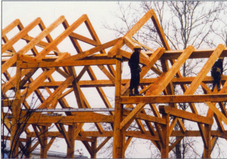
Workers help Lancaster County Timber Frames erect a barn at the Plain & Fancy restaurant in Bird-in-Hand.
